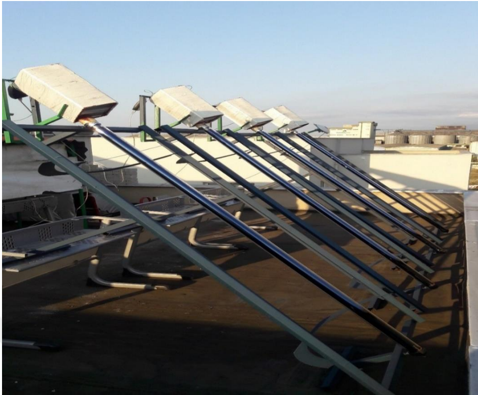
Figure 3.8. Photograph showing the heat pipes receives solar radiation at an angle of 41^\circ .
