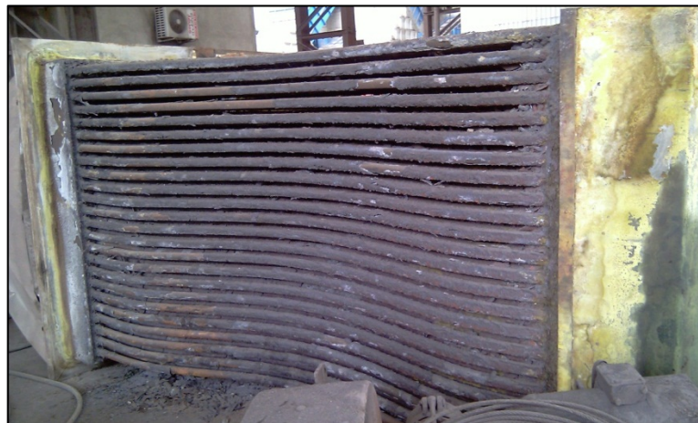
c) Destroyed recuperator.
