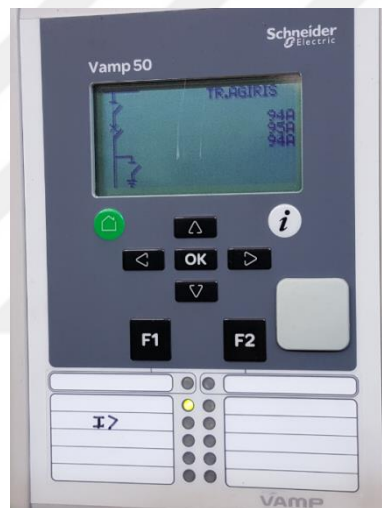
Figure 3.11. Phase-earth protection relay.
