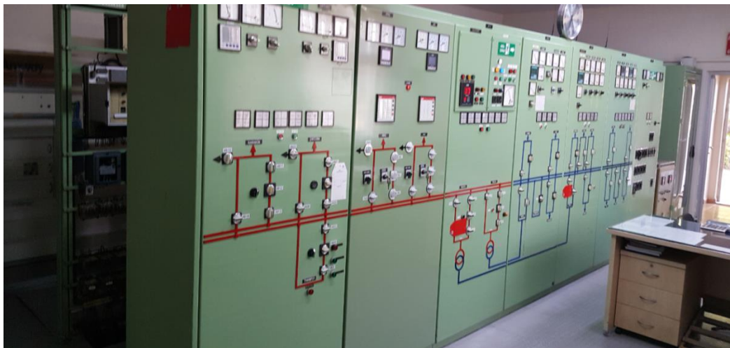
Figure 4.2. Safranbolu substation control room.
