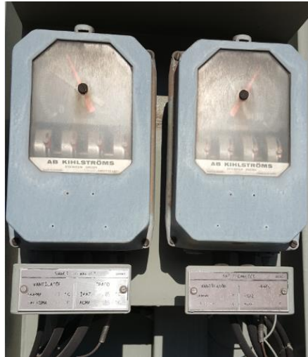
Figure 3.12. Transformer's oil and winding temperature protection relays.
