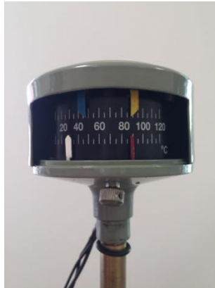
Figure 3.13. Tank temperature protection relay.
