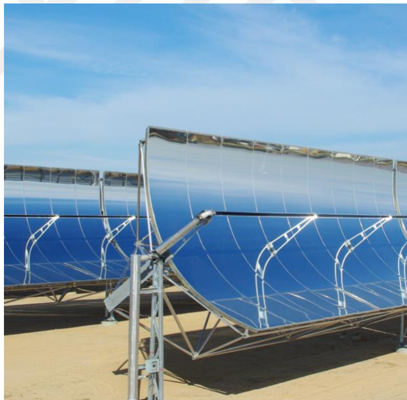
Figure 4.2. SkyFuel parabolic trough collectors [4].
