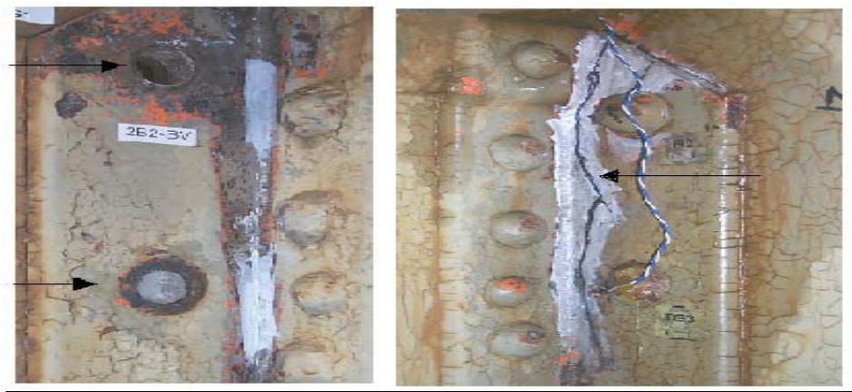
Figure 2.10. Examples of fatigue damage in riveted stringer-to-floor-beam connections [28,29].
