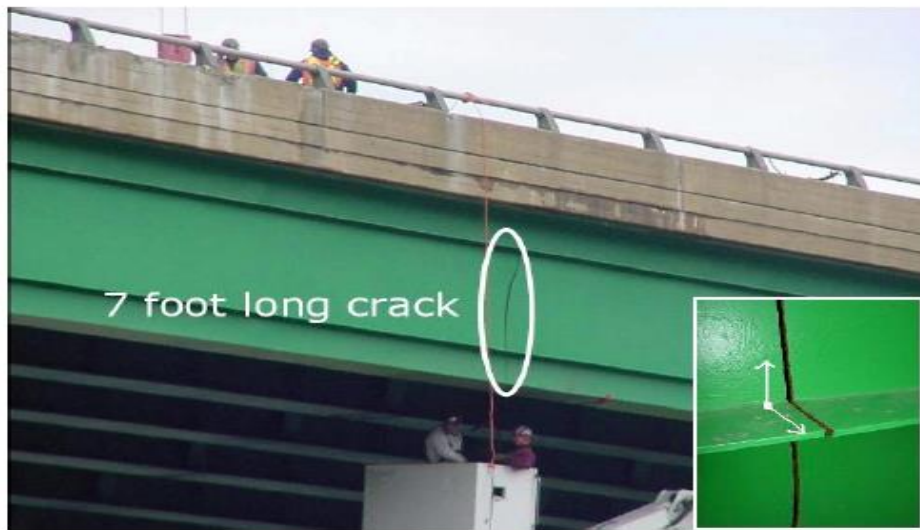
Figure 2.9. Cracking in a bridge girder starting from weld defects at a weld intersection point [33].
