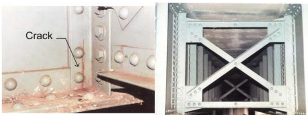
Figure 2.10. Fatigue cracking in the riveted connection of cross-bracing elements.
