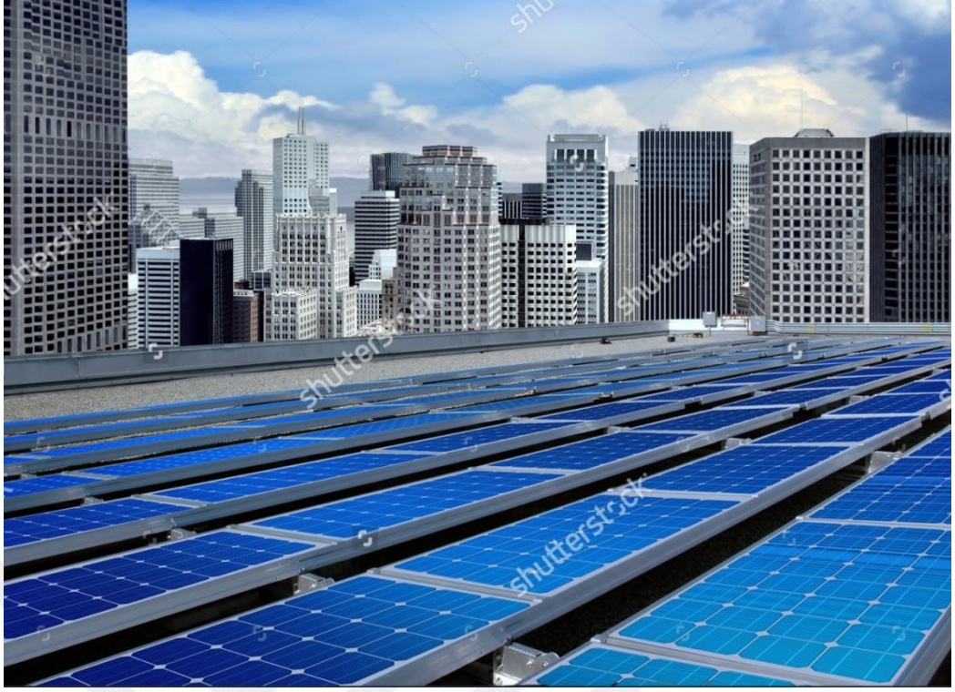
Şekil 3.16. Güneş kolektörleri ( http://image.shutterstock.com/z/stock-photo-solar-panels-on-the-roof-of-modern-skyscraper-61502710.jpg )
