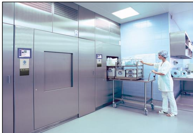
Figure 4.9: Example of a clean area with autoclave machines
