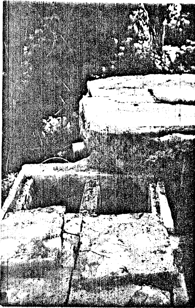
Figure 3.4 (c) Photograph of the Inlet View of the Channels
