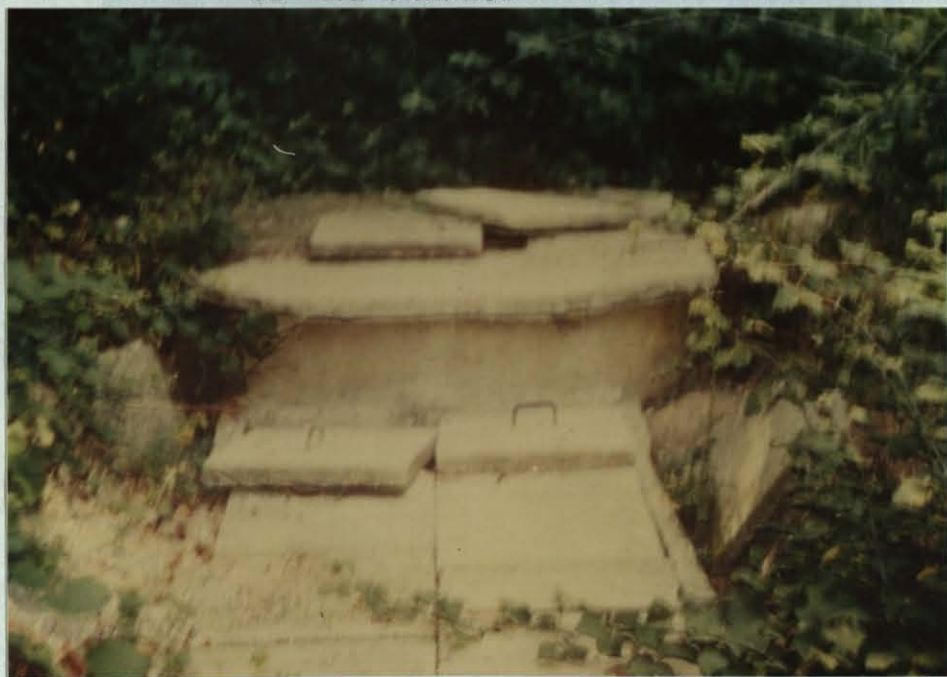
Figure 12 : Photograph of the Outlet Tank (Final Tank)
