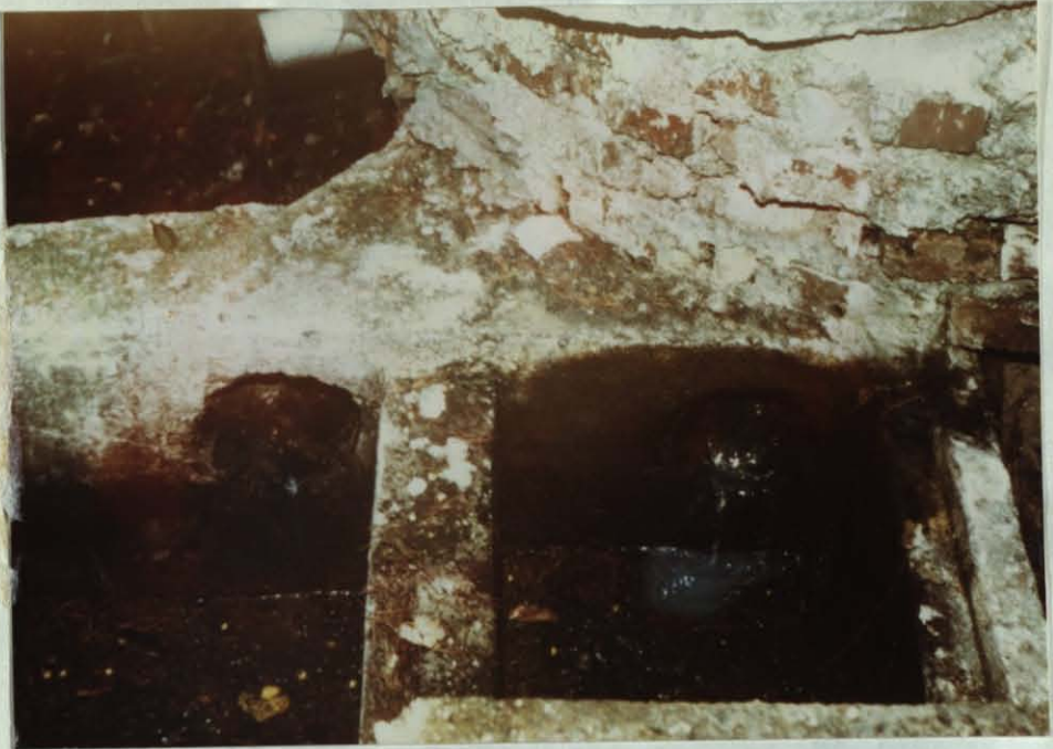
Figure 8: Photograph of the Inlets
