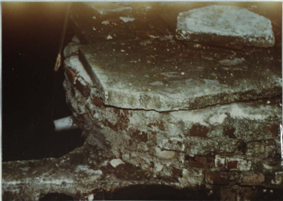
Figure 7 : Photograph of the Inlet Tank "L" Type Covering Plate and Overflow pipe
