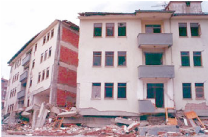
Figure 3.26 The basements are collapsed while the other floors are healthy
