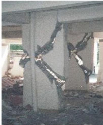
Figure 3.29 Very dangerous crackes on the columns of building.
