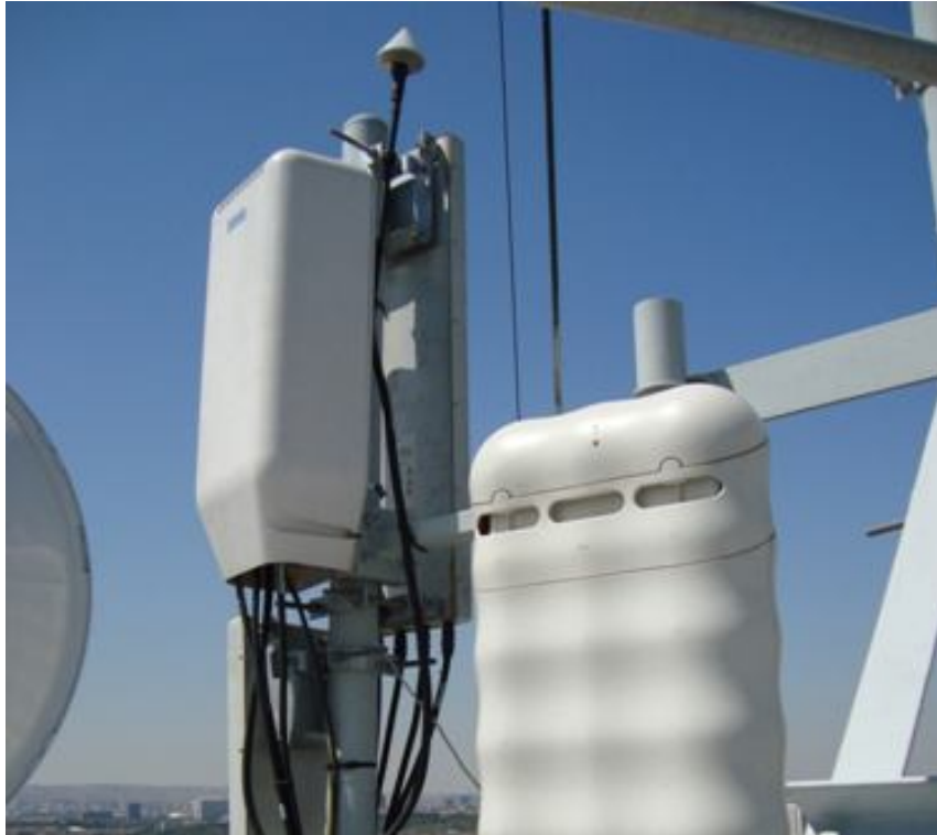
Figure 6.13: WiMAX Base Station 2
