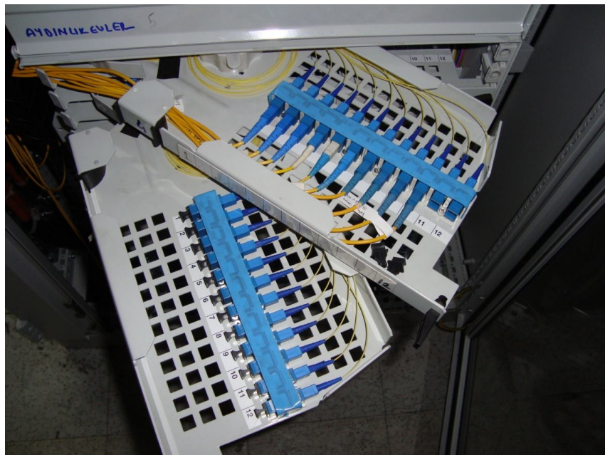
Figure 6.14: Optical Distribution Frame (ODF)
