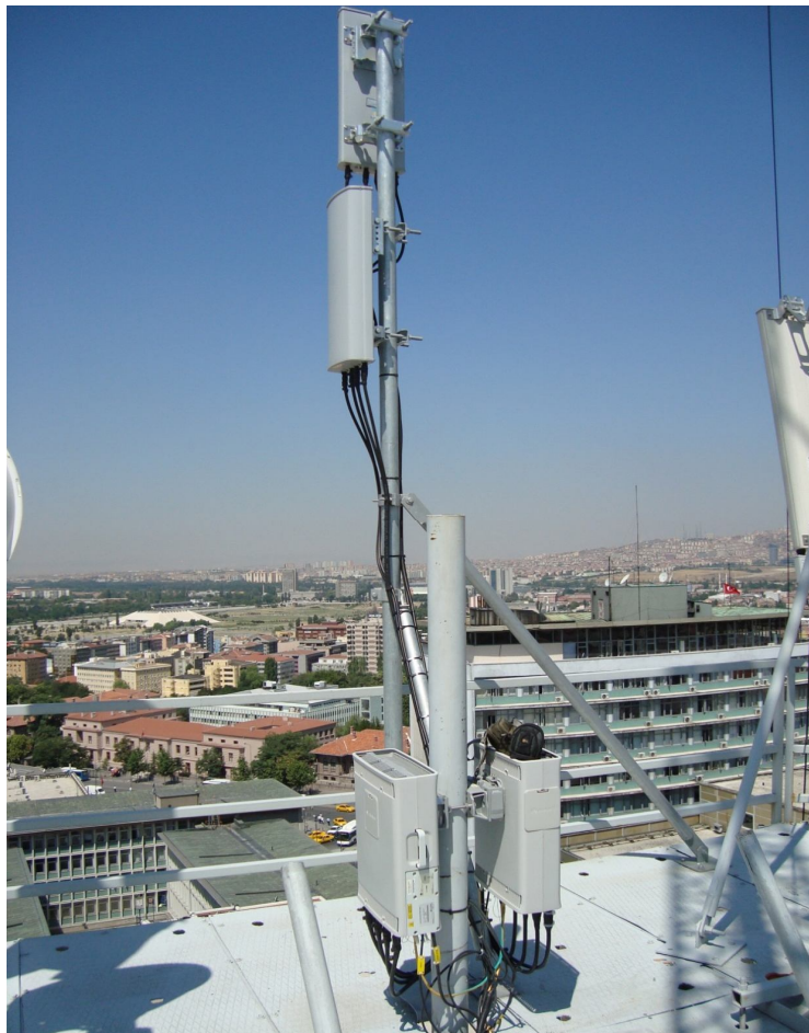
Figure 6.12: WiMAX Base Station 1
