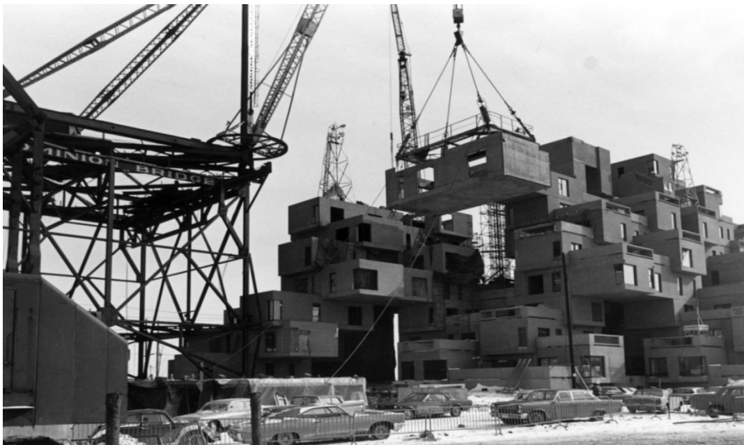
Figure 16. Construction process of Habitat 67. Modules inserted one by one to complete the whole building [80]
