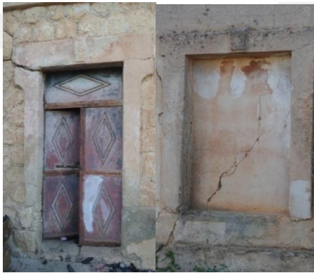
Figure 59. Show the door and window without a change in the Italian style
