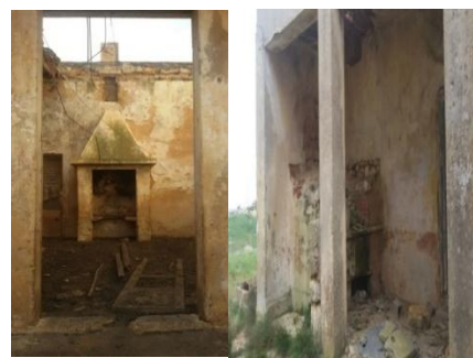
Figure 76. Showing heating inside the house and also in the back separately
