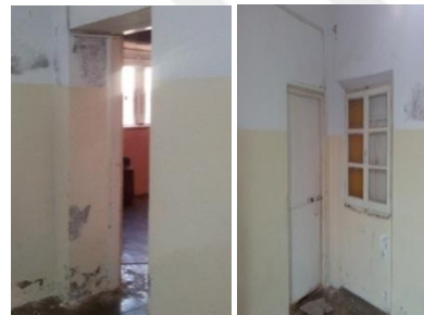
Figure 33. Show the door and the window from the inside with the width of the wall
