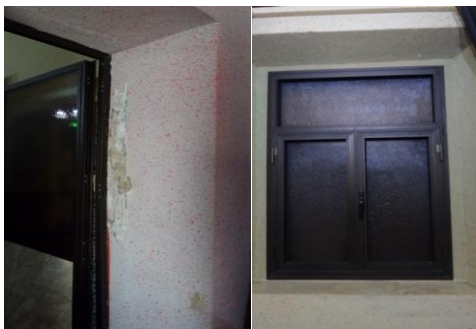
Figure 21. Shows the door and the window from the inside, which shows the width of the wall
