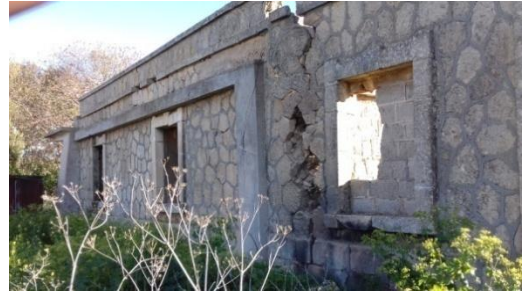
Figure 65. Showing the right side of the house with the windows also cracked the wall
