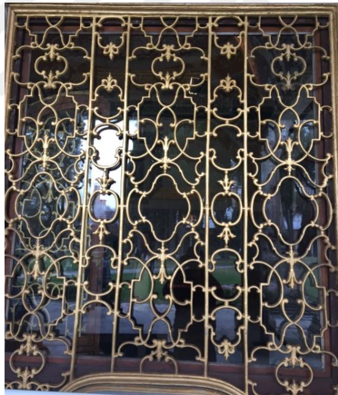
Figure A7: Topkapi Palace – Divan - Window protection - Metal forms installed in front of the glass window
