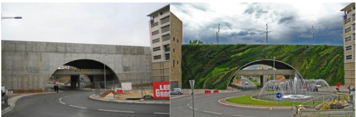
Figure 2.22: Vertical garden installation on bridge sides (Timur & Karaca, 2013)
