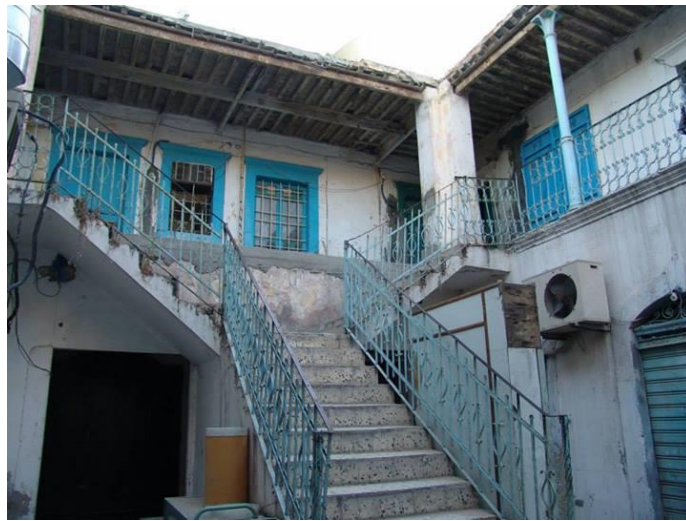
Figure 4.8: A house in Tripoli castle with the addition of inappropriate material and utilities. (Author's collection)
