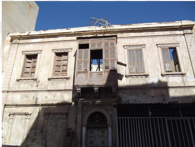
Figure 2.18: A front view of a house in Tripoli castle that has not been rehabilitated (Author's collection)
