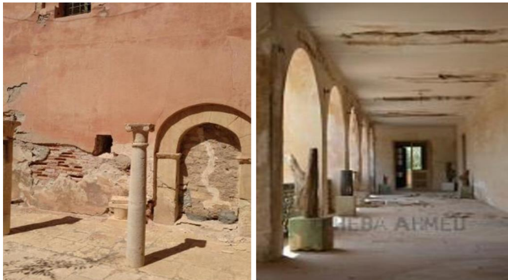
Figure 4.2: Deep cracks in the walls and slabs of Red Saraya. (Author's collection)
