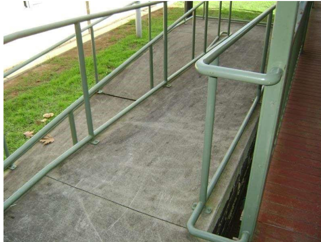
Figure 2.17: Good ramp example with handrails on both sides and floor is finished with non-slippery material (Fidzani, et al., 2013)
