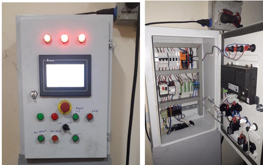
Figure 24: Electric Control Panel
