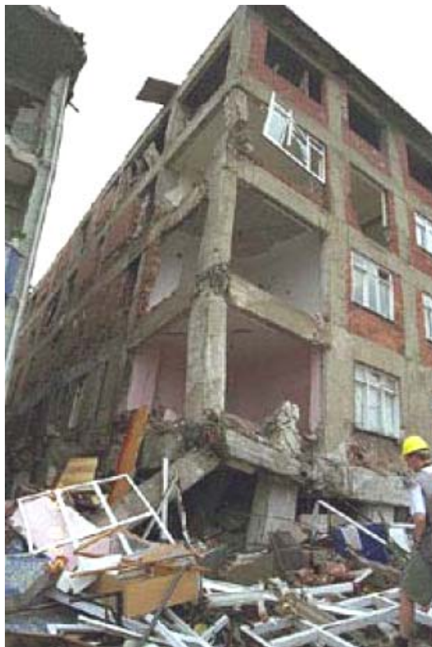
Figure 2.1. Damage on beam-column joint during Kocaeli EQ (Sezen et al. , 2000)
