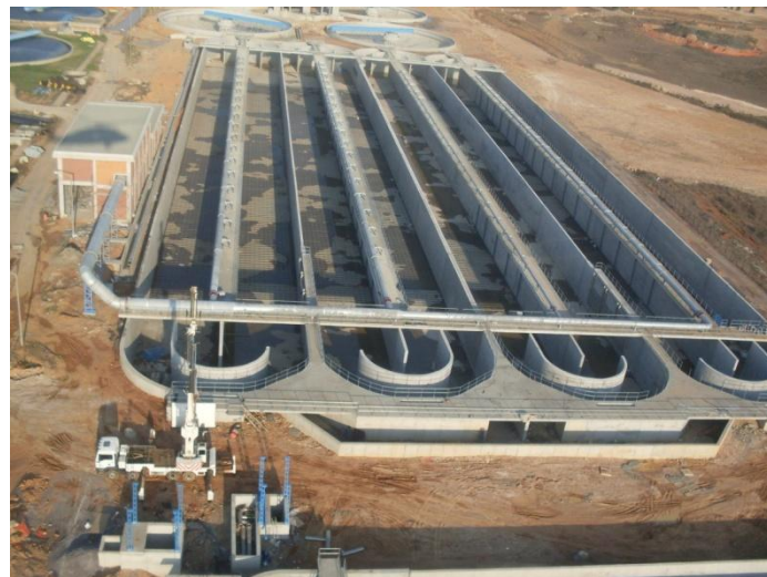
Figure 3.9. Aeration Tanks of Paşaköy WWTP
