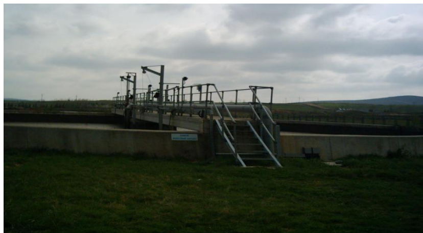
Figure 3.15. Sludge Storage Tank of Paşaköy WWTP
