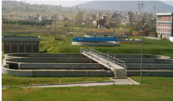
Figure 3.7. Bio-P Tanks of Paşaköy WWTTP
