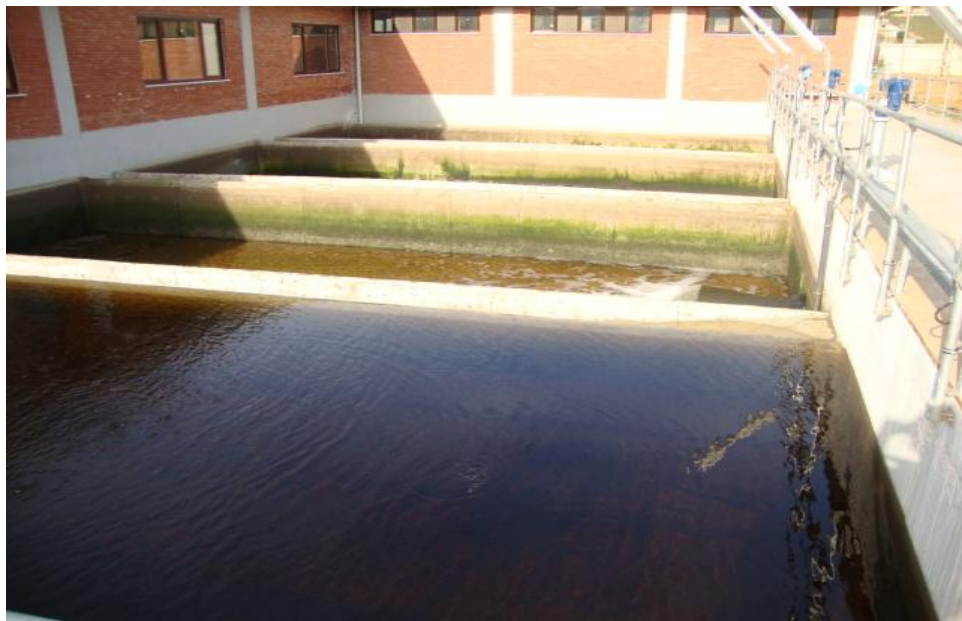
Figure 3.14. Sand Filters of Paşaköy WWTP
