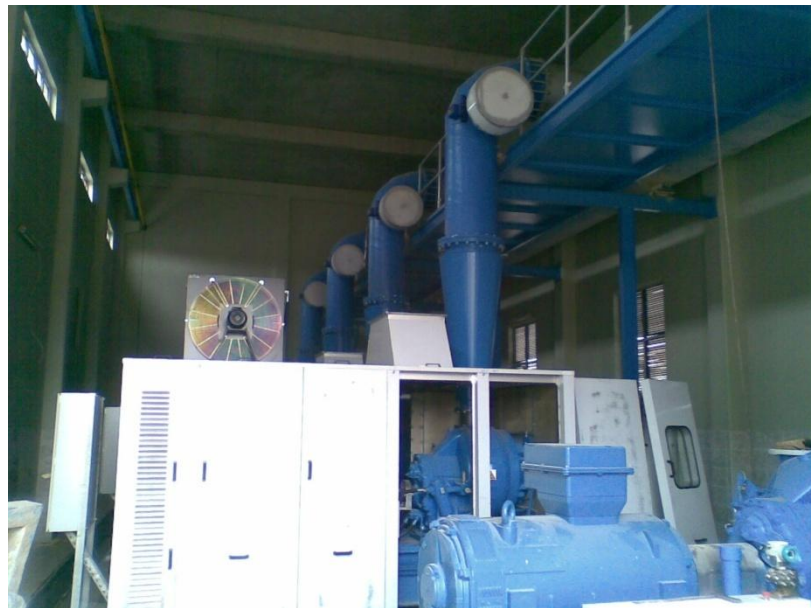
Figure 3.11. Blower Building of Paşaköy WWTP
