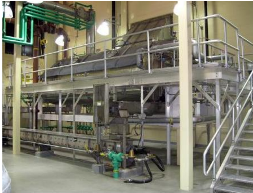
Figure 3.17. Sludge Drying Unit of Paşaköy WWTP
