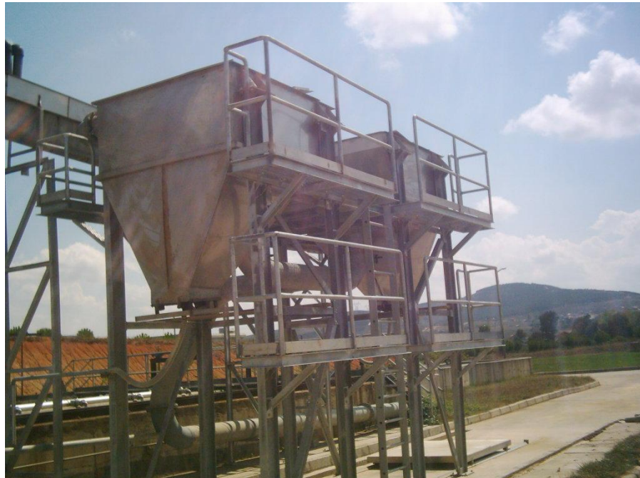
Figure 3.6. Grit Separation of Paşaköy WWTP
