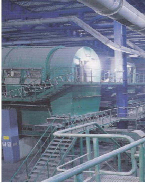
Figure 7.14. Kemberburgaz Compost Facility (İSTAÇ, 2010)
