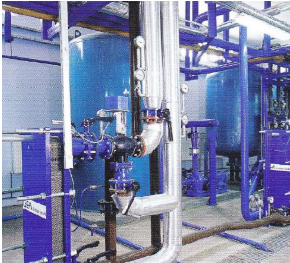
Figure 7.10. Heat Exchanger (İSTAÇ, 2010)
