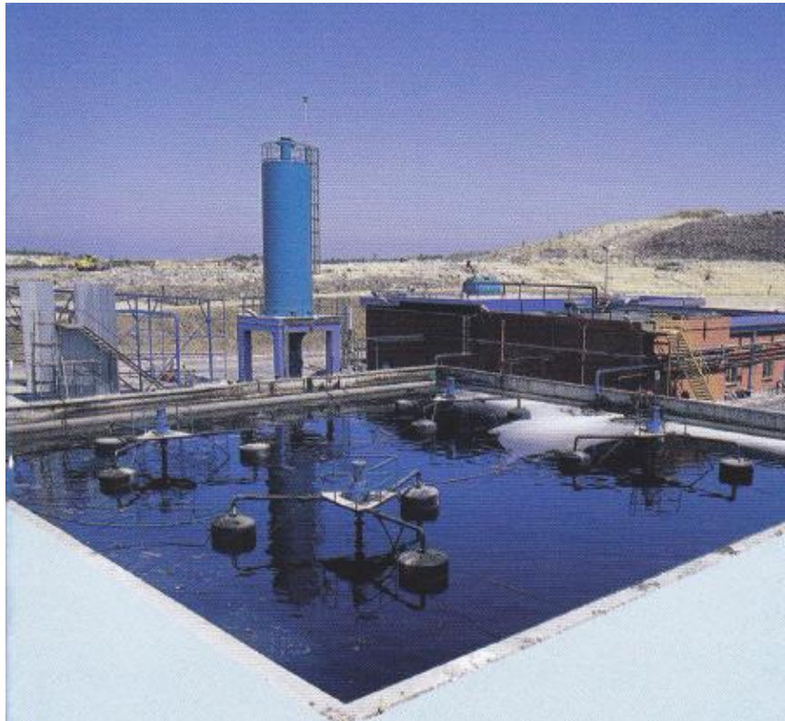
Figure 7.8. Sedimentation pool (İSTAÇ, 2010)
