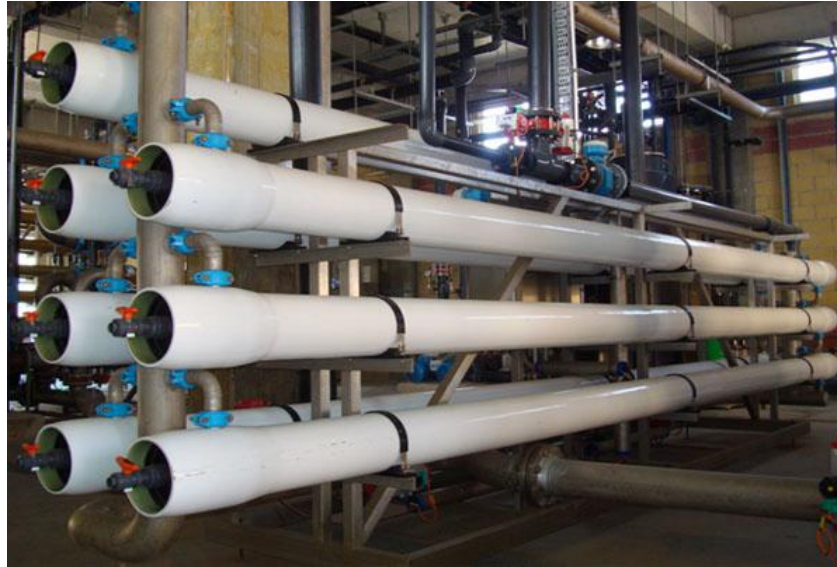
Figure 7.12. Nano filtration capillary membranes (İSTAÇ, 2010)
