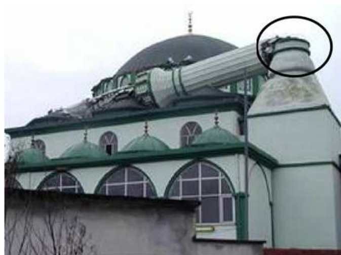
Figure 5.3. Collapse of minaret on its main building. [5]
