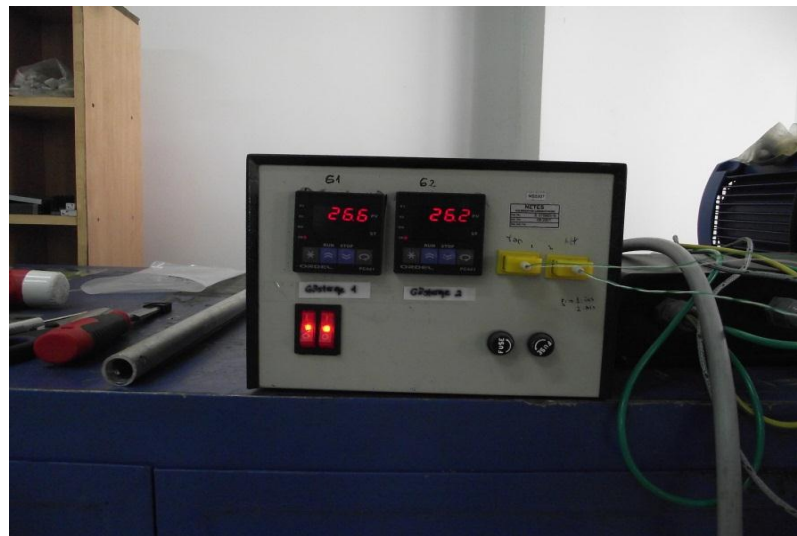
Figure 4.3. Temperature control unit.
