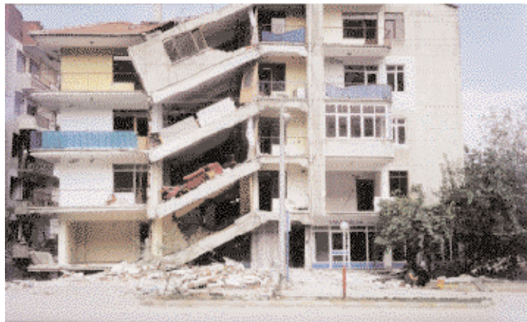
Figure 1.3. Earthquake induced progressive collapse from Kocaeli, Turkey (RMS, 1999).
