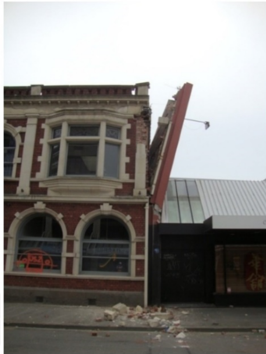
Figure 2.3. Out-of-plane instability of the wall subjected to face load due to a lack of ties between the face-loaded wall and rest of the structure [17].
