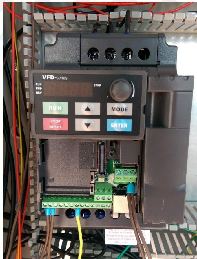
Figure 3.6. Variable frequency driver of the pump.
