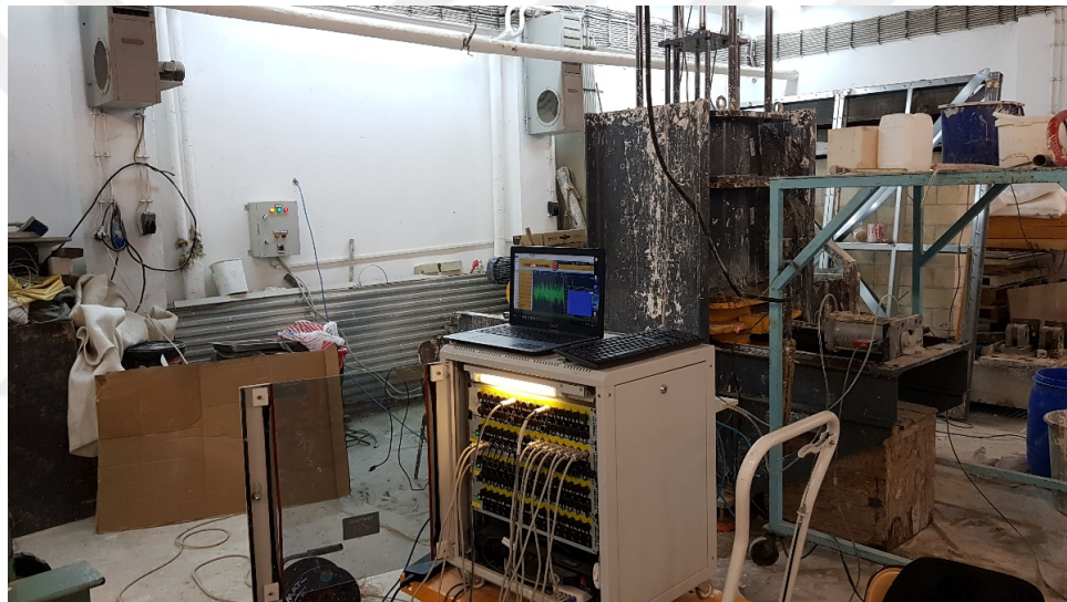
Figure 3.13. 112 Channel Data Logger with the UCSD.
