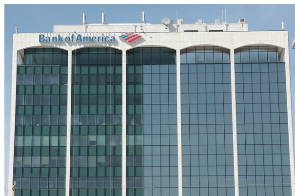
Figure 2.62: Bank of America during installation of scratch resistant, exterior window film from Madico. The right side of the building has the new film installed, Florida.
