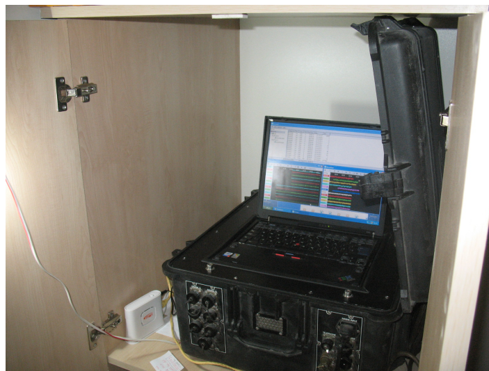
Figure 3.10. Data acquisition system, located in the cabinet for safety
