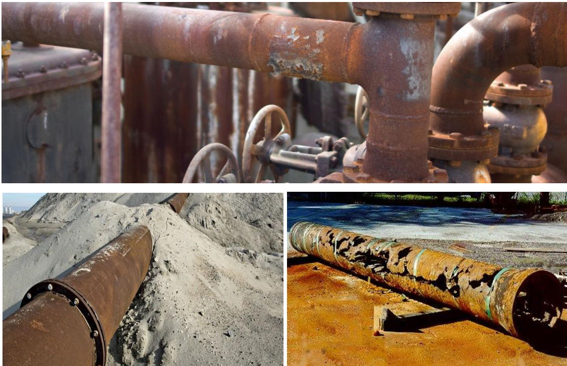
Figure 1.2. Examples of observable corrosion condition at CPS Desalator.
