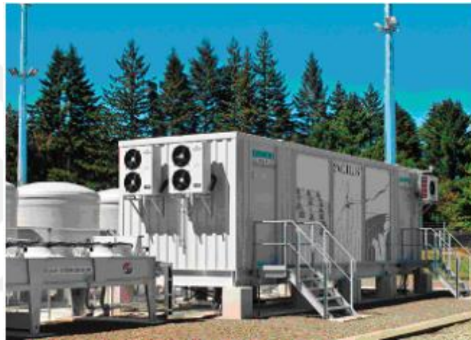
Figure 5.40 One of the two SVC PLUS units at Kikiwa, New Zealand
