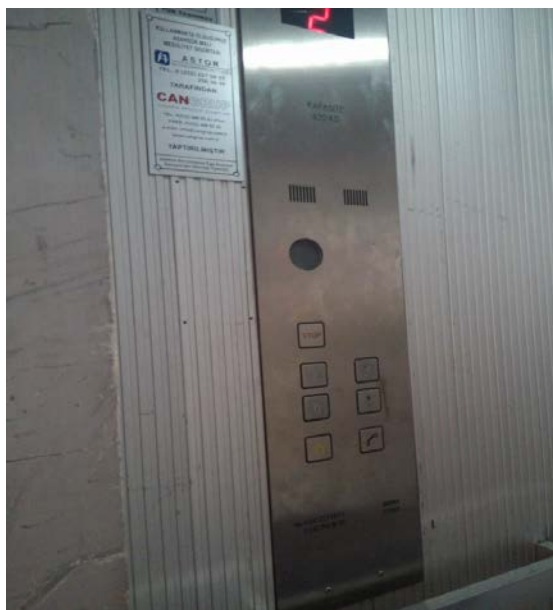
Figure 15: The Control Panel of the Elevator
