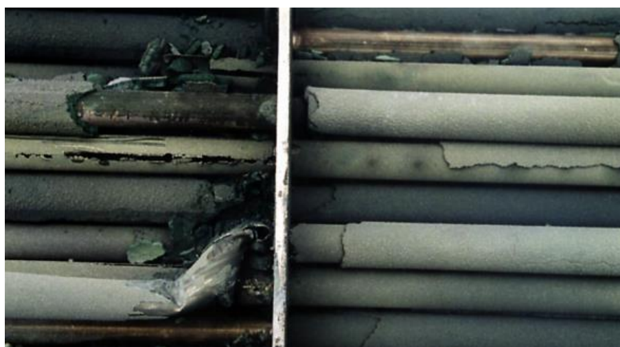
Figure 1.3. Deposit-covered and corroded rich/lean amine exchanger tubes
