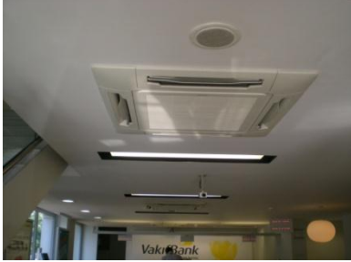
Figure 4.66. Vakıf Bank Izmir branch ceiling ventilation system
