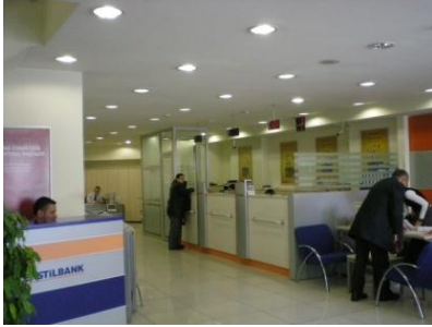
Figure 4.13. Textile bank ceiling lighting system
