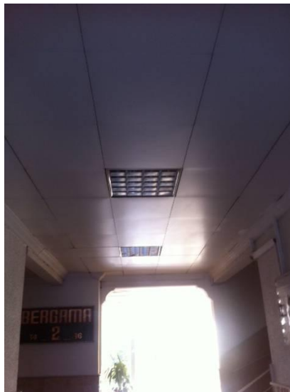
Figure 4.38 LED Lighting at Atakent Bostanli
