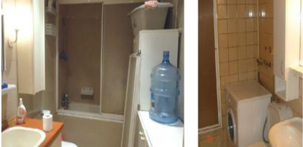
Figure 4.6 Foccets and showers installed in Etap Konutlari
