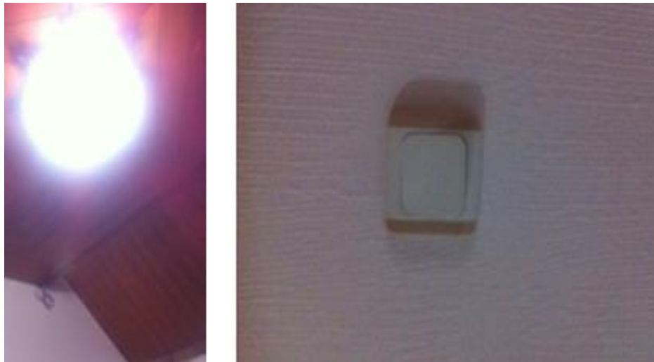
Figure 4.21 Lighting Equipment and Bulb at Mert Kule
