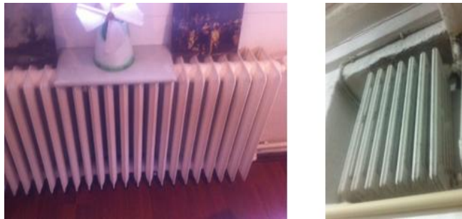
Figure 4.18 Unit Heating Equipment at Mert Kule
