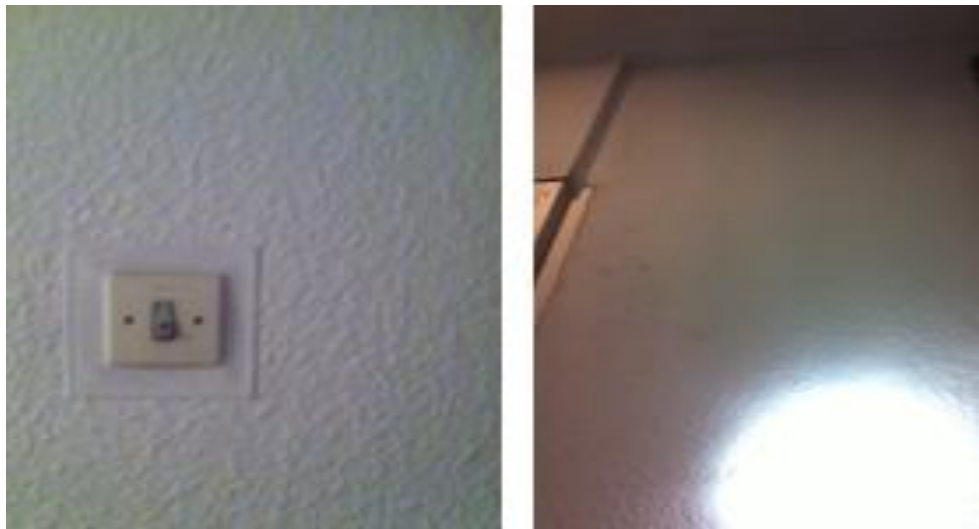
Figure 4.13 Lighting Switches at Etap Konutlari
