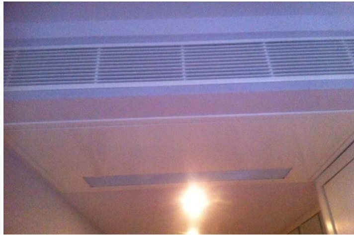
Figure 4.96 Cooling System is designed aesthetically
