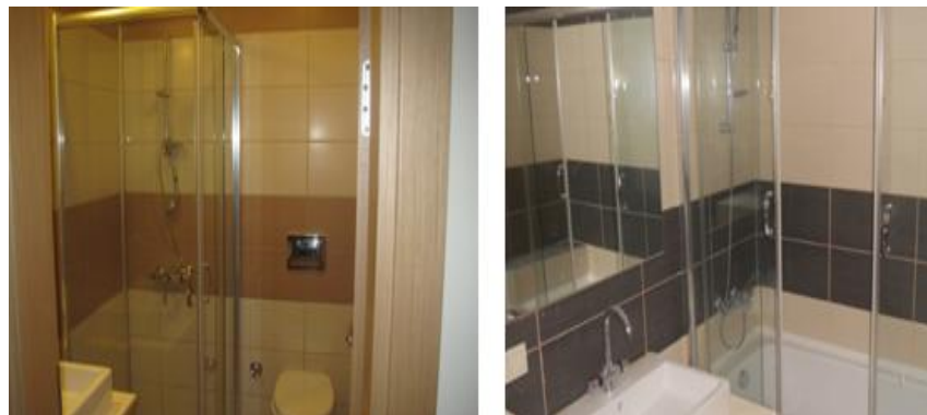
Figure 4.116 Bathroom Equipments to save water at Metrokent
