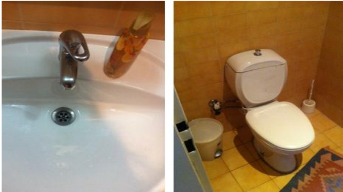
Figure 4.54 Water Fixtures of units
