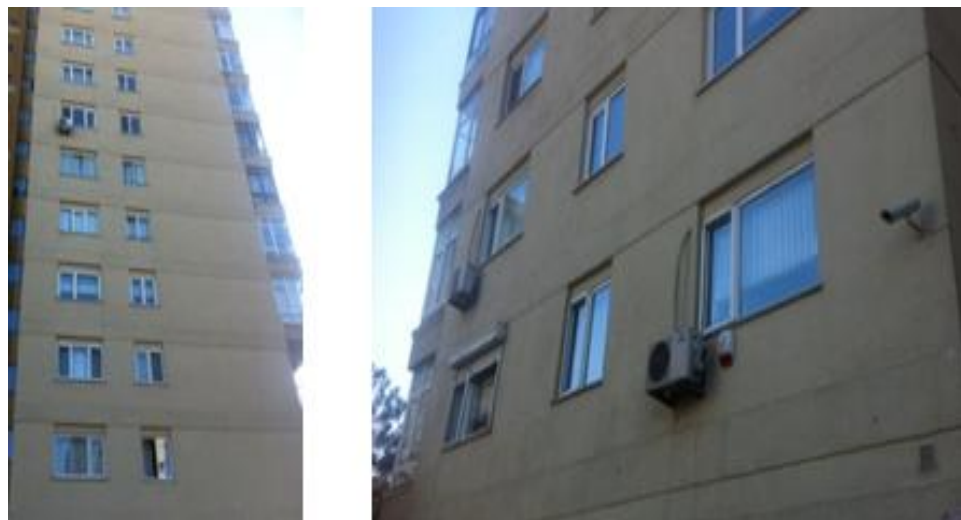
Figure 4.19 Outside AC units at Mert Kule
