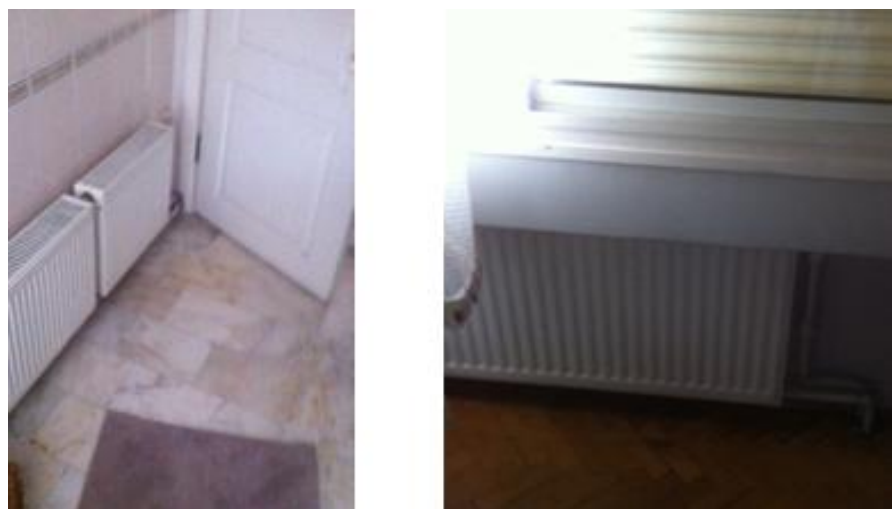
Figure 4.79 Heating Fixtures at Pamukkale Konutlari
