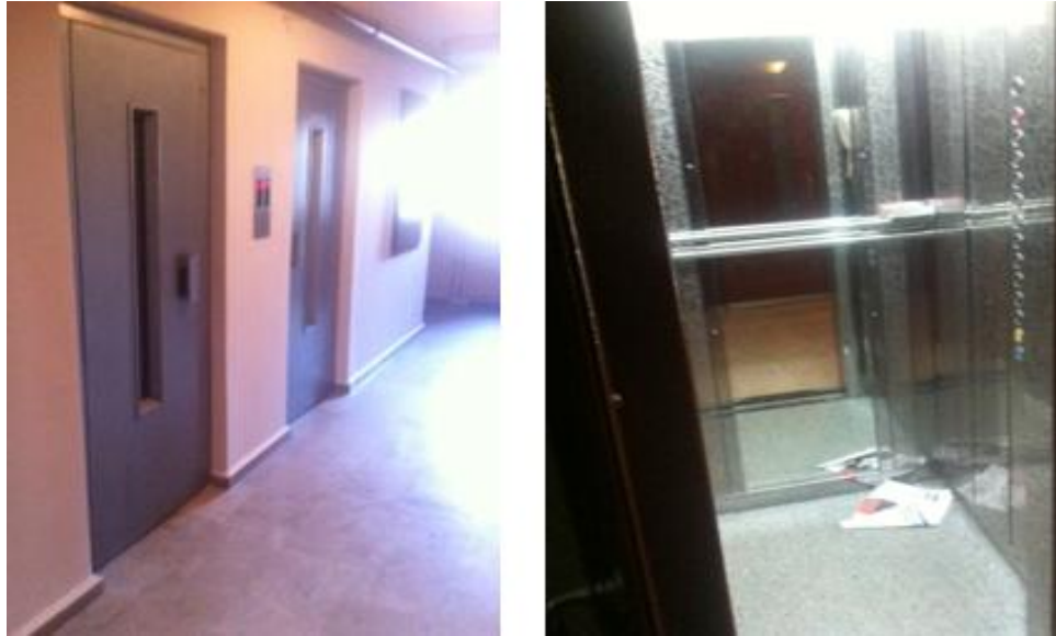
Figure 4.62 Elevator entrance from the lobby of Blok A Tercuman Sitesi
