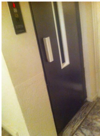
Figure 4.47 Elevator Doors at Atakent Bostanli
