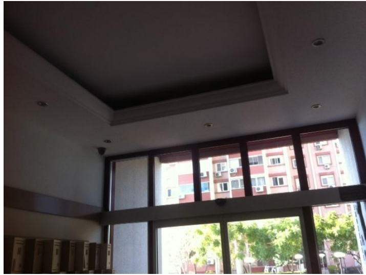
Figure 4.82 Spot Lights at the entrance of Pamukkale Konutlari
