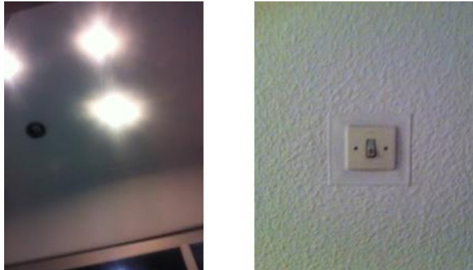
Figure 4.5 Common Apartment Lighting at Etap Konutlari
