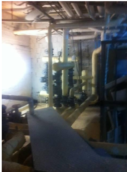
Figure 4.17 Heating Control Room at Mert Kule
