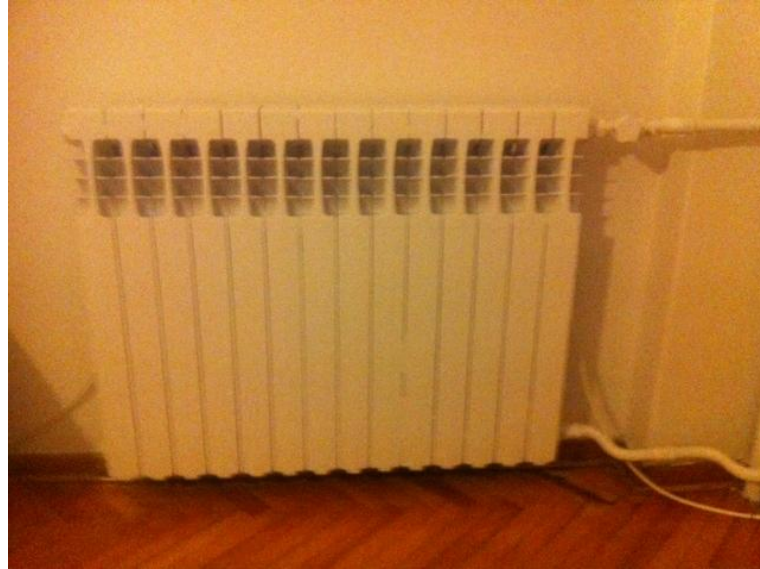
Figure 4.50 Heating System in the units at Tercuman Sitesi
