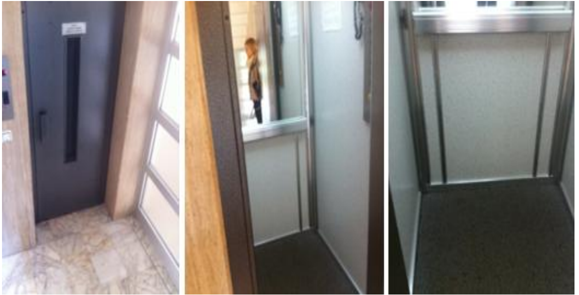
Figure 4.76 Elevators at Sepas Sitesi
