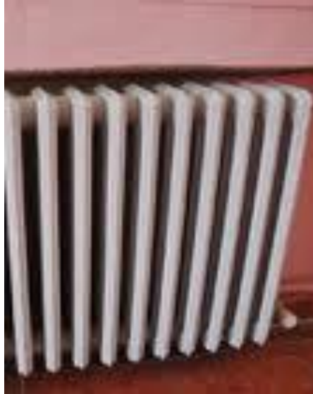
Figure 4.35 Heating Fixtures at Atakent Bostanli
