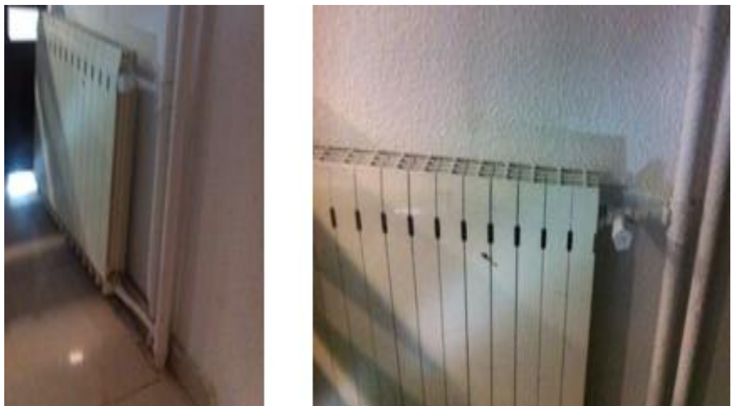
Figure 4.2 Heating Fixtures at Ataköy Etap Konutlari
