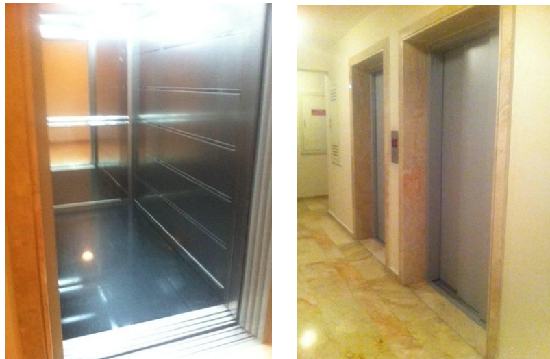
Figure 4.143 Elevators at Mavisehir
