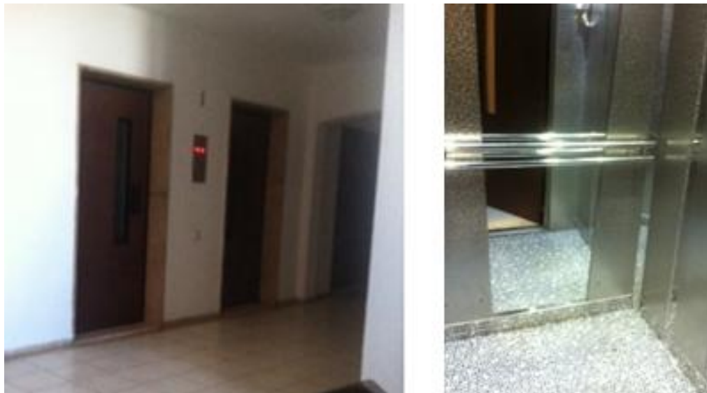
Figure 4.92 Elevators at the Building at Mavisehir Konutlari
