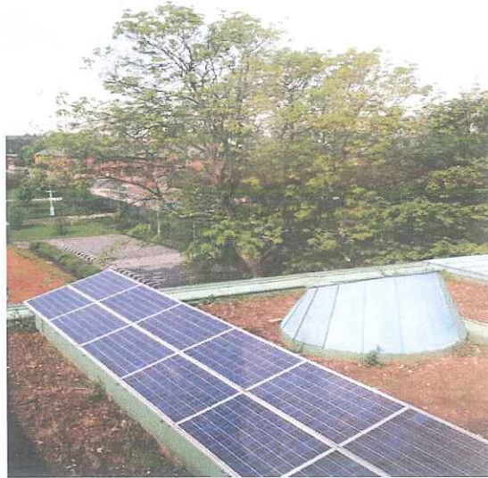
Figure 4.9. Assisi St. Francis Academy, Photovoltaic Panel
