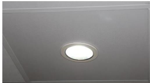
Figure 4.25. Private Ata Saglık-Ceiling Luminaires
