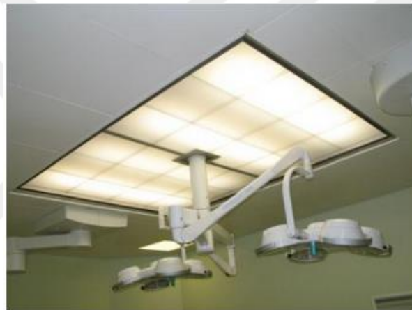
Figure 3.6. General and Local Lighting in Operation Rooms
