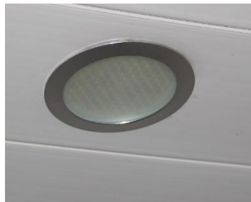
Figure 4.78. Private Gazi Hospital-Bathroom Ceiling Luminaire
