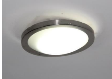
Figure 4.74. Private Gazi Hospital-Ceiling Luminaires
