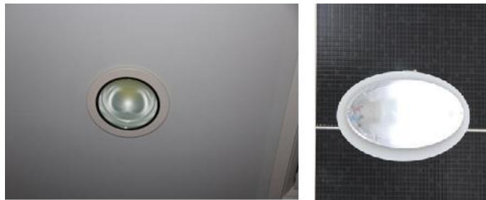
Figure 4.29. Private Ata Saglık-Bathroom Ceiling and Wall Mounted Luminaire
