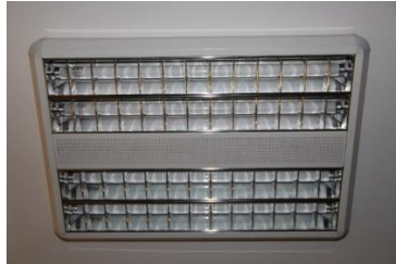
Figure 4.56. Private Su Hospital-Ceiling Luminaire
