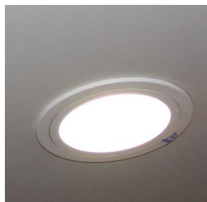
Figure 4.62. Private Su Hospital-Bathroom Ceiling Luminaire
