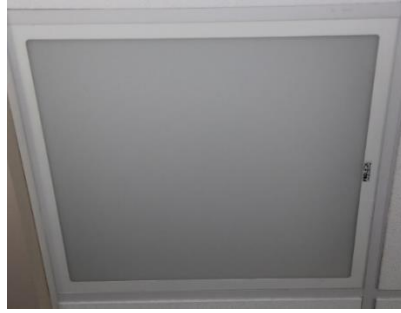
Figure 4.4. Private Tmaztepe Hospital-Ceiling Luminaires
