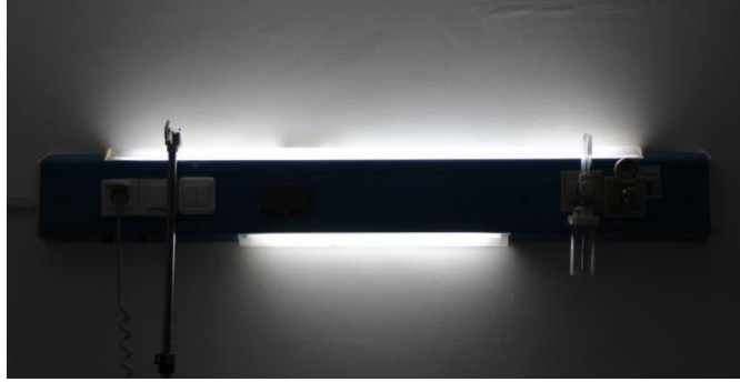
Figure 4.76. Private Gazi Hospital-Direct and Indirect Luminaires
