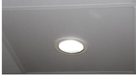
Figure 4.6. Private Tmaztepe Hospital-Entrance Ceiling Luminaire
