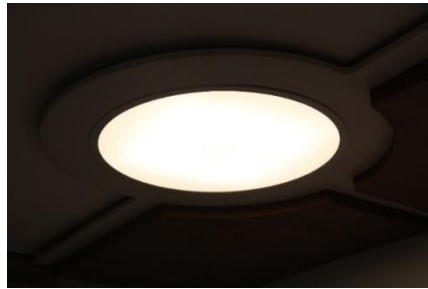
Figure 4.88. Private Karatas Hospital-Ceiling Luminaire
