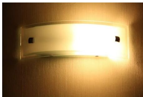
Figure 4.60. Private Su Hospital-Wall Mounted Luminaires
