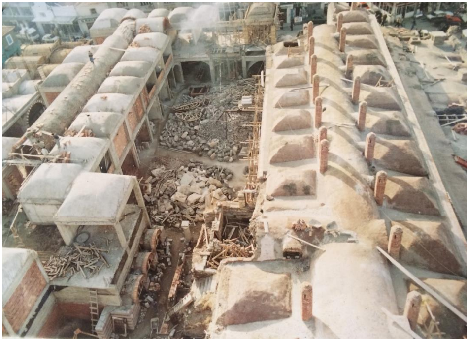
Figure 4.12. Kızlarağası Inn, the view of courtyard during renovation (between 1988 and 1993) (Kızlarağası Archive, 2016)
