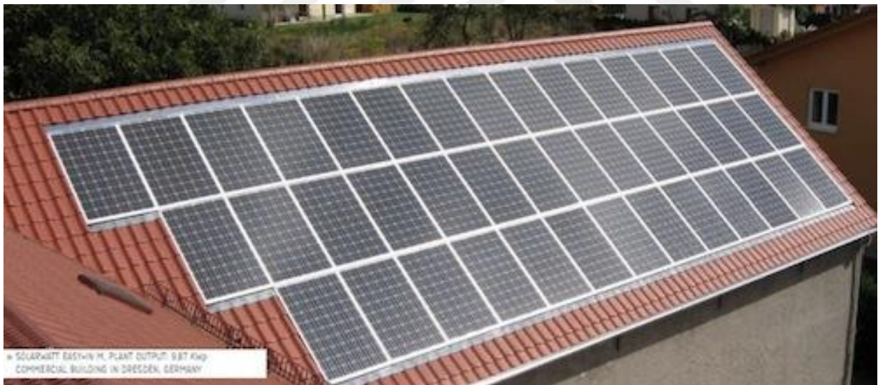
Figure 3.21 BIPV Roof fixation of Solar panels on a commercial building in Germany
