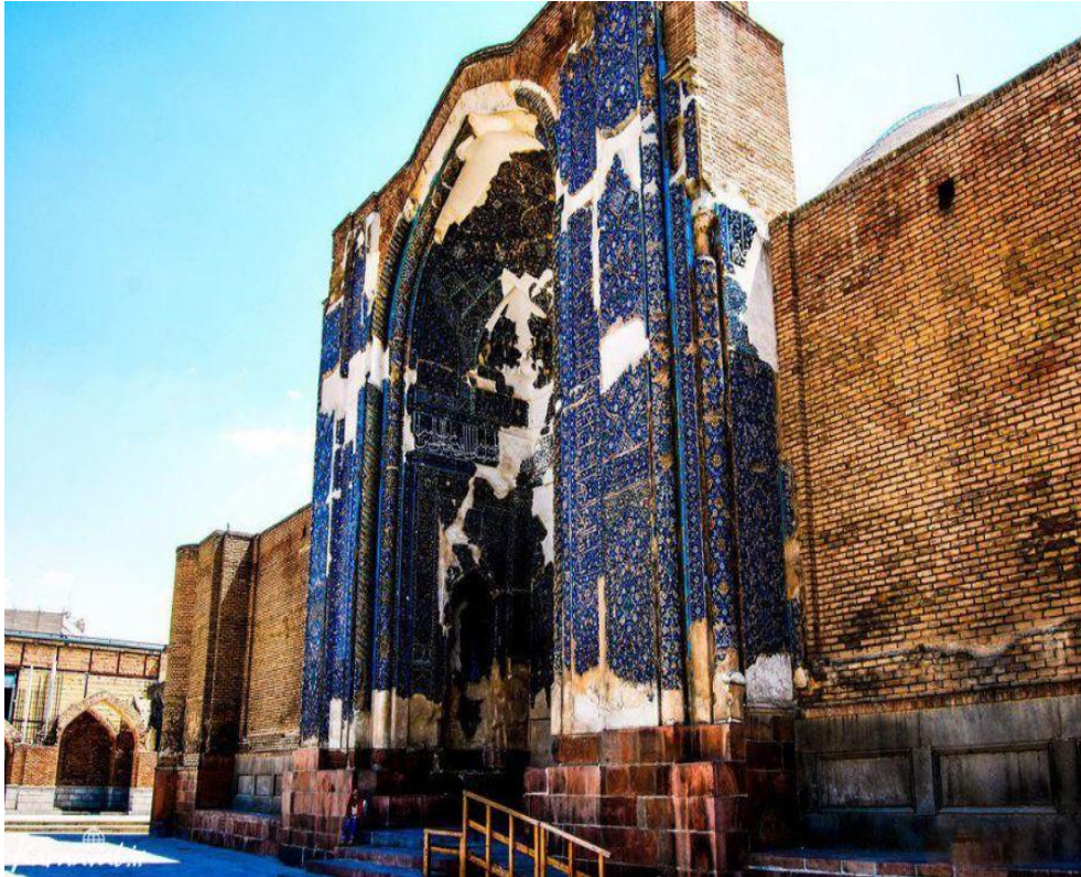
Figure 2.24. Tabriz Blue Mosque (1351-1469), Entrance, 14th World Conference on Earthquake Engineering . (Photography by Saide Khali Safa)
