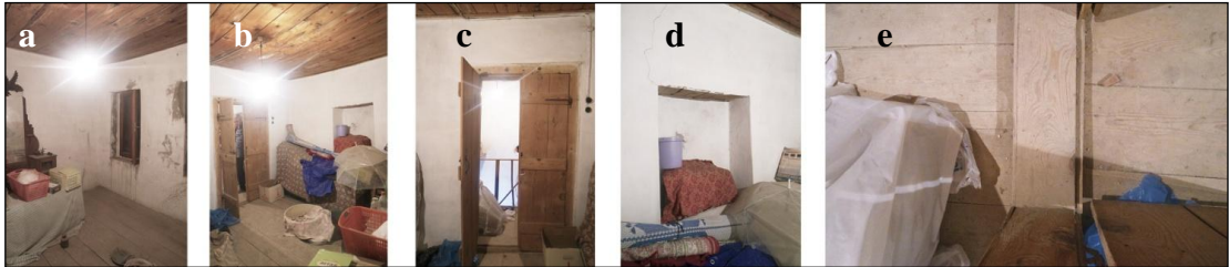
Figure 4.23. First Floor a. Room2; b. Room (H); c.,d.,e. Door with two wings, alcove and wooden floor details (S.Sevimbige archive, 2017)
