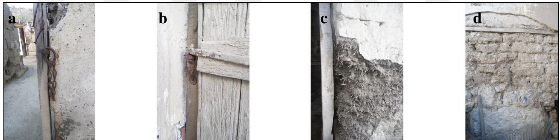
Figure 4.31. Mustafa Orşahin's House a., b. courtyard door details; c.,d. adobe wall and bonding timber system (S.Sevimbige archive, 2017)
