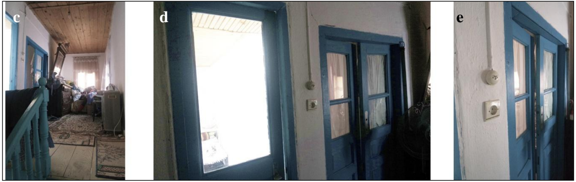
First floor c. hall; d.,e. bedroom doors and electric switch details (S.Sevimbige archive, 2017)
