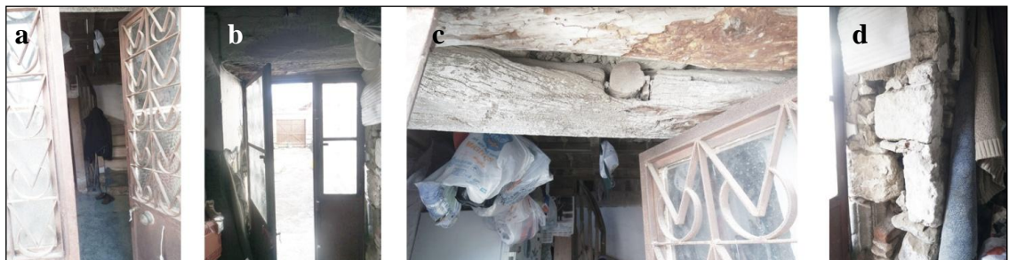
Figure 4.32. Mustafa Orşahin's House ground floor a., b., c., d. Entrance door and ceiling - wall details (View F) (S.Sevimbige archive, 2017)
