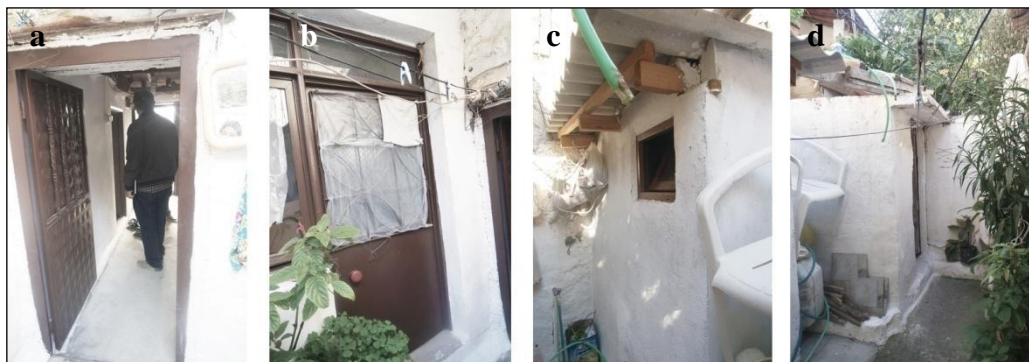
Figure 4.19. Bahise Sakallıoğlu House ground floor a. Exit door to courtyard; b. Entrance of additional room in; c.,d. Warehouse and toilet in the courtyard (S.Sevimbige archive, 2017)
