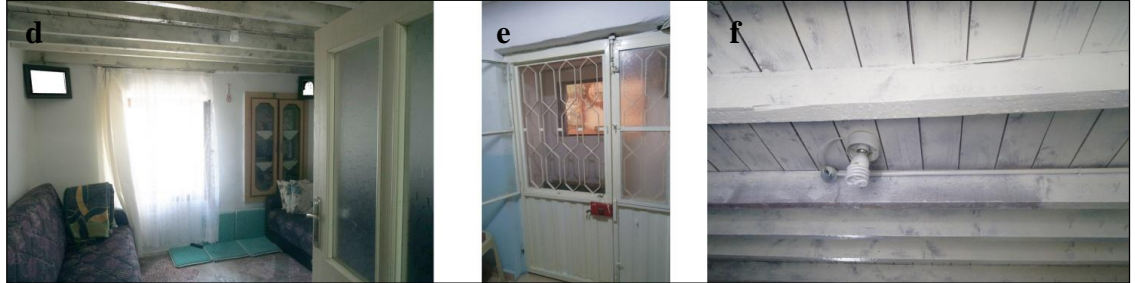
d. Ground floor living room; e. Ground floor former entrance door; f. ceiling (S.Sevimbige archive, 2017)
