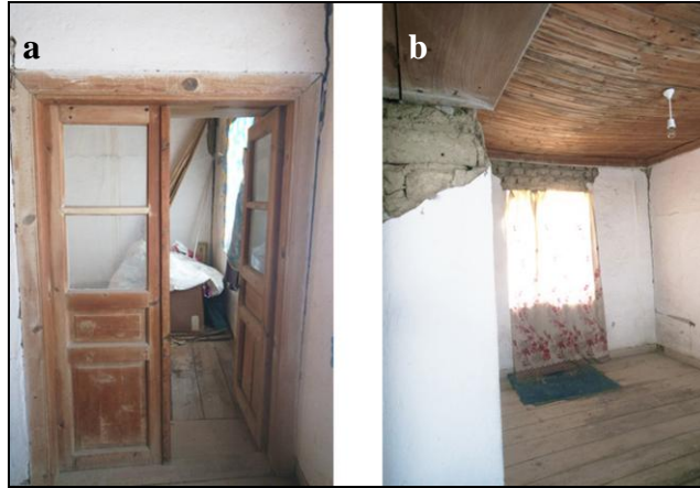
Figure 4.34. Mustafa Orşahin's House first floor a. Room entrance (H); b. Roof (S.Sevimbige archive, 2017)
