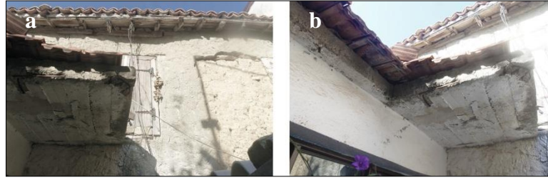
Figure 4.20. Bahise Sakallioğlu House e., f. View of the upper floor wall containing "haney" from the courtyard and roof details (*haney: parts of the house between the floors, hall) (S.Sevimbige archive, 2017)
