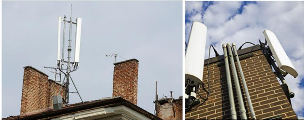
Figure 1.5: Base Station on Roof (Alamy, 2010)
