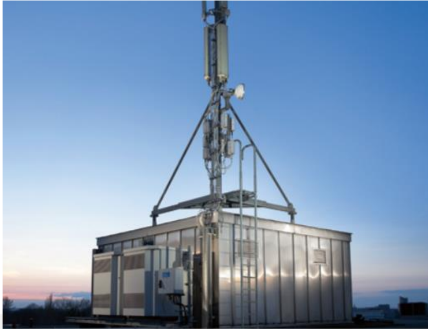
Figure 1.6: Base Station Cabins (KUARK, 2013)
