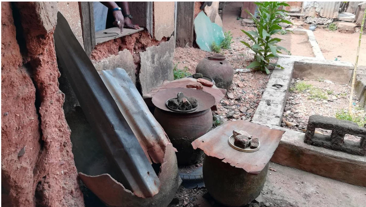
Figure 4.15. Deteriorated Structural Elements
