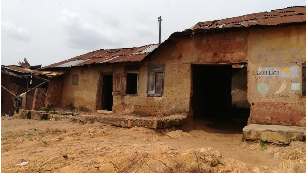
Figure 4.14. Structural Elements Washed Away by Erosion Water
