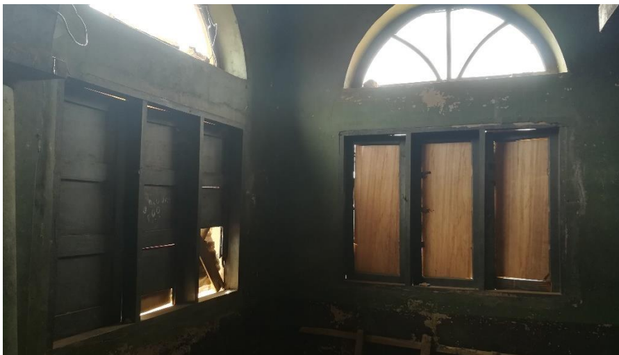
Figure 4.4. Washing away of the interior by entrance of rain water
