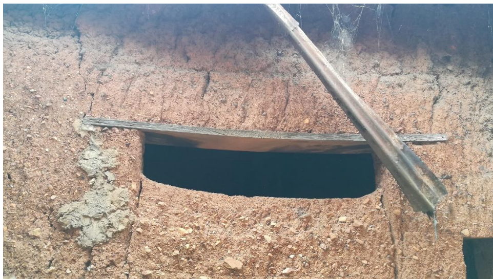
Figure 4.1. Effect of heat on wall plastering, Aare Latoosa Palace
