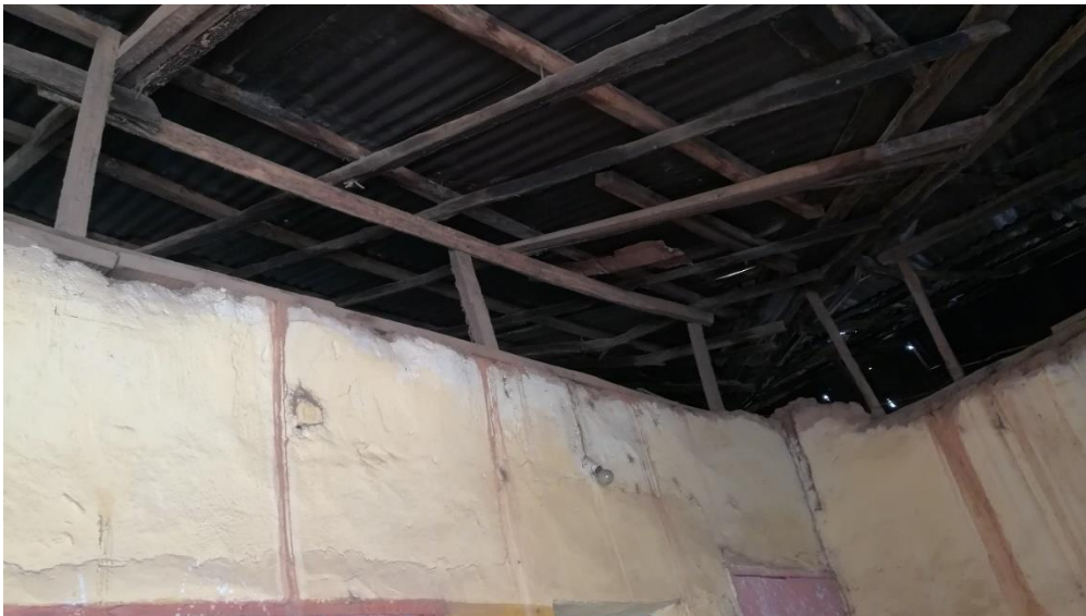
Figure 4.2. Deterioration of interior by water, Aare Latosa Palace
