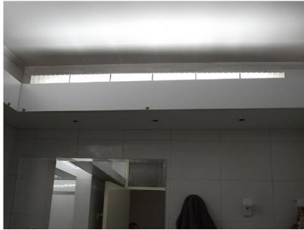
A: Bathroom lighting
