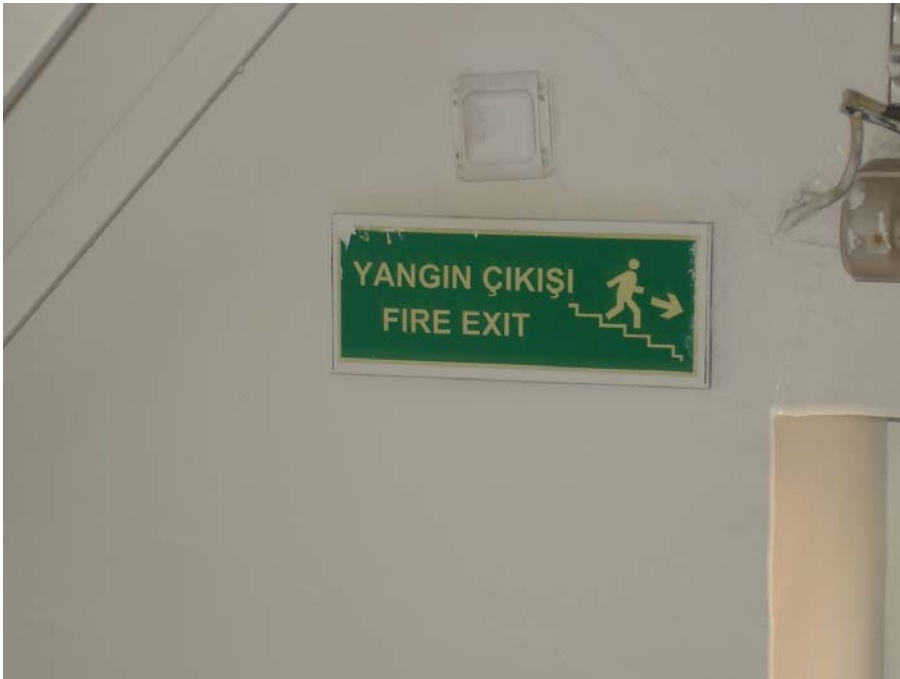
Figure A4.7. A view of directional sign (the fire exit).
