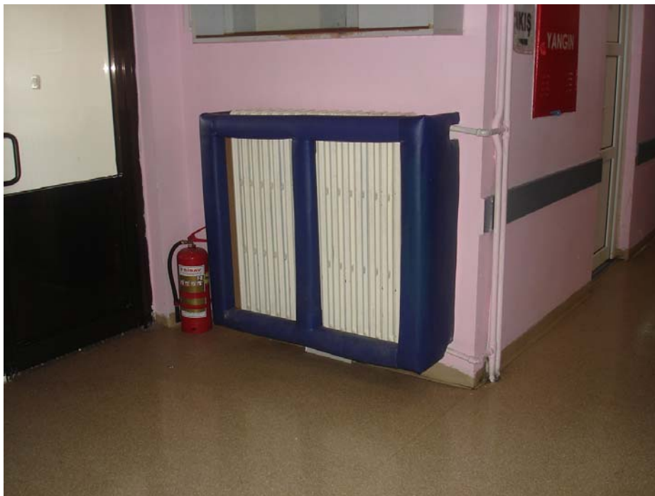
Figure A4.9. A view of radiators.
