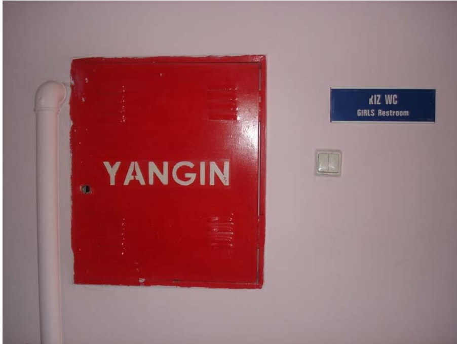
Figure A4.8. A view of situation object identification sign (the fire box).
