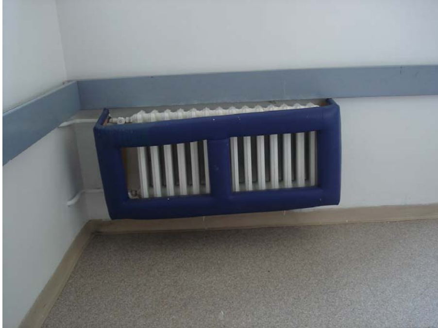
Figure A4.10. A view of radiators.
