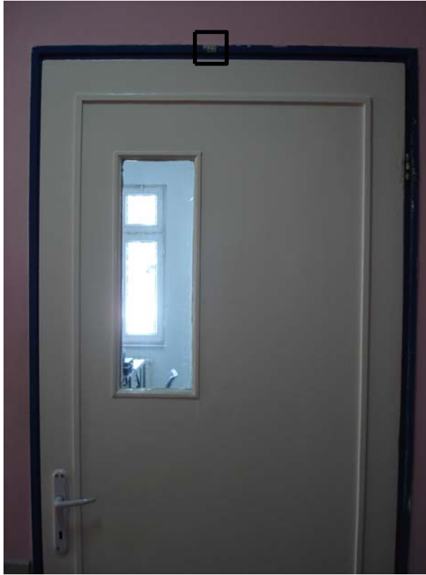
Figure A4.1. A view of destination identification sign (door number) on the door frame on top and the middle.
