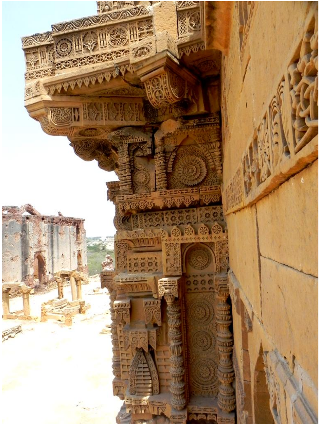
Figure 4.28: Side view of the balcony ensemble on the west façade, Tomb of Jam Nizam. (Taken by the author)
