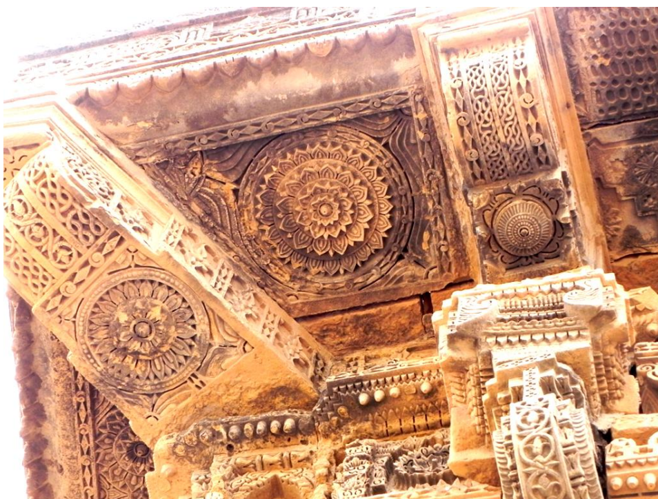
Figure 4.27: Close-up of supporting brackets, balcony ensemble on the west façade, Tomb of Jam Nizam. (Taken by the author)
