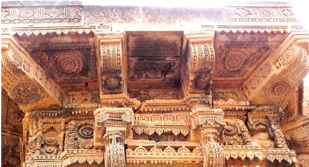
Figure 4.26: View of under surface of projecting balcony and supporting brackets, balcony ensemble on the west façade, Tomb of Jam Nizam. (Taken by the author)
