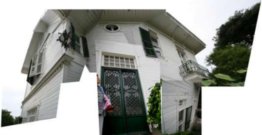
Photo 4.3.64 Collage showing the north elevation, see the side entrance that opens directly to the staircase
