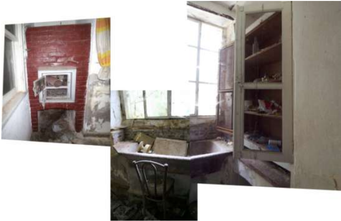
Photo 4.3.97 Right across the stairs, there is the stove and the laundry, the sash window on the left and the cupboard on the right.
