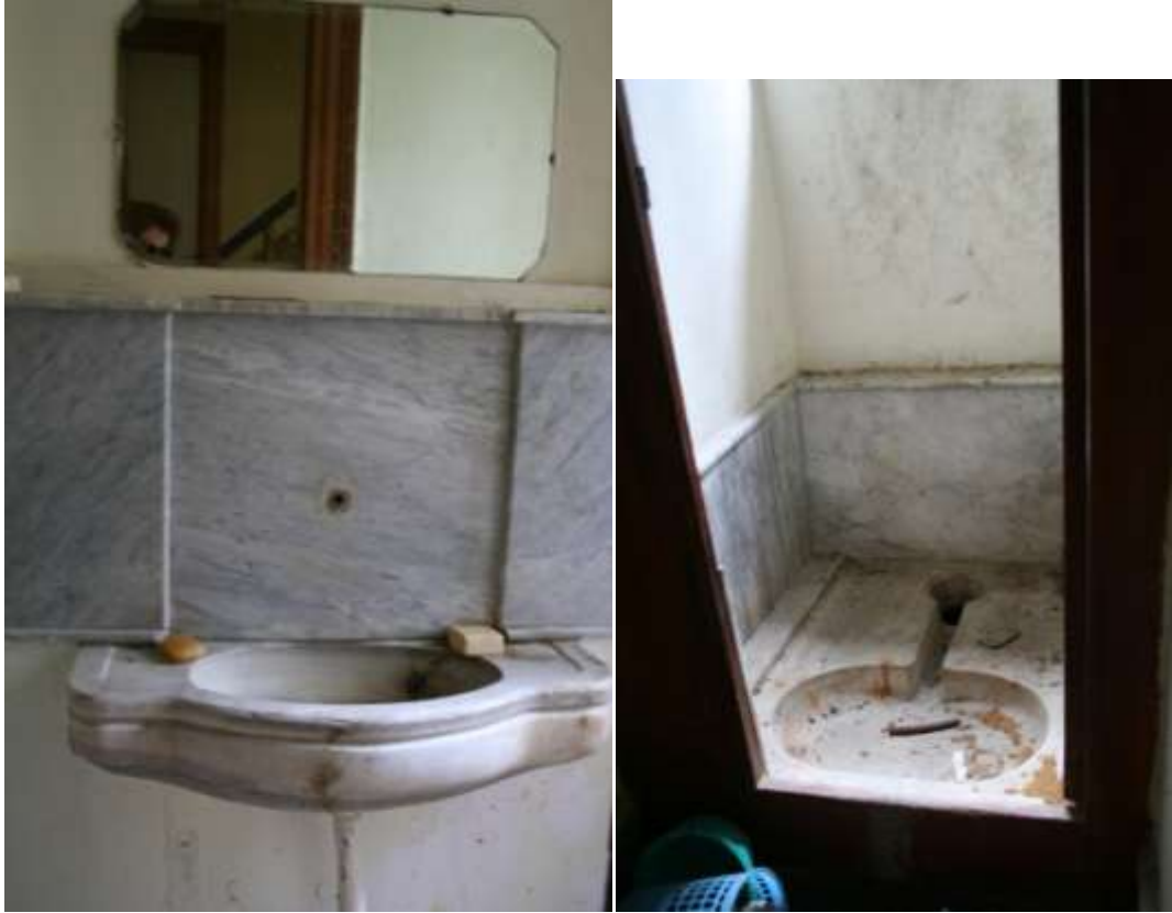
Photo 4.3.95 Marble wash basin and toilet in the entrance floor
