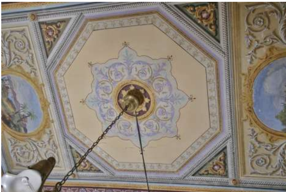
Photo 4.3.110 The ceiling of the room on the front-right side (Photo by Teo)
