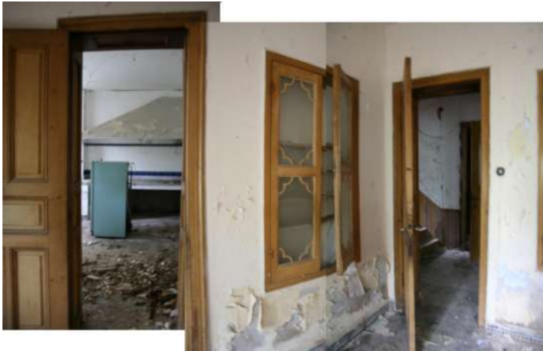
Photo 4.3.99 The multifunction living room on the ground floor, for casual gatherings, for sewing, dining, etc...
