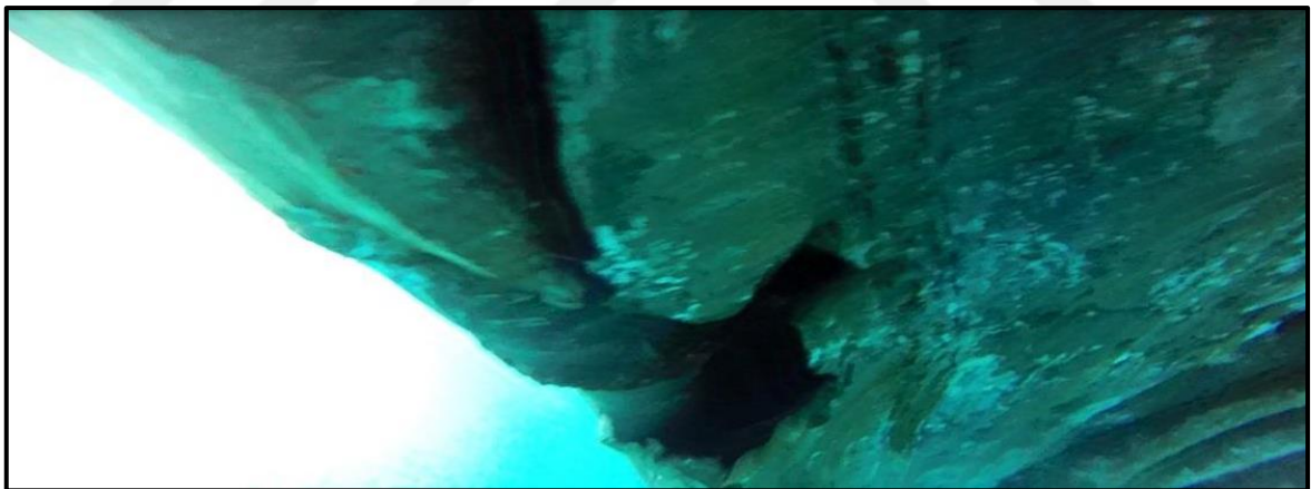
Figure 7.6. Damaged Parts as Recorded by the Diver's Camera (The Accident Investigation Report, 2017).
