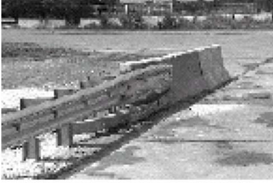
VERTICAL FLARED BACK TRANSITION DAMAGE
